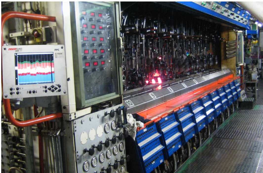
Fig. 1 PPC System at a AIS 10 Section
